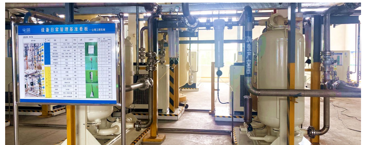
Air-pressure system post retrofitting as part of the joint energy-saving project with public works of Sinochem High Performance Fiber
