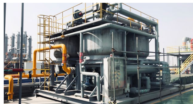
Yangnong Ruiheng exhaust gas adsorption equipment for chlorobenzene production
