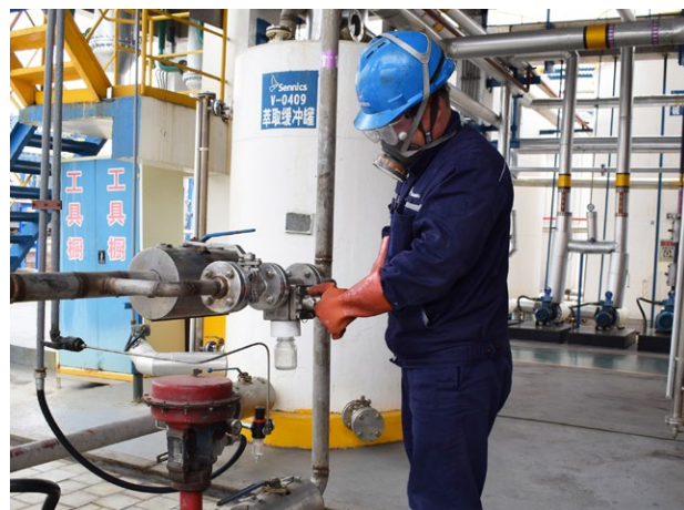
Shandong Huahong has installed flanged sampling valves on its process pipeline and tank openings to reduce risks to staff performing sampling work
