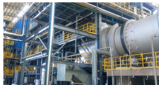
Yangnong Ruitai hazardous waste incineration
